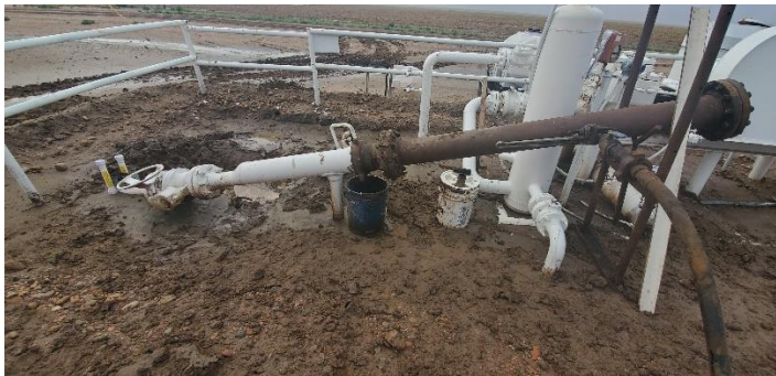
Figure 7--Temporary Extension to Launcher Trap with Piping to Push Product Behind the ILI Tool
