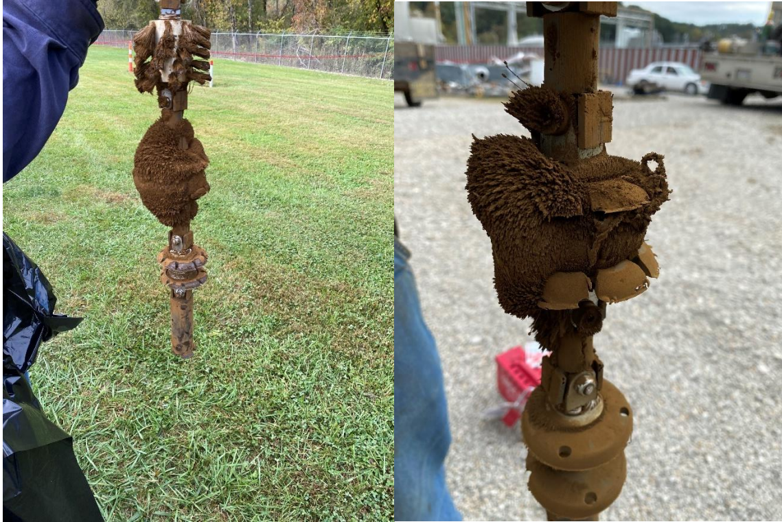
Figure 20--Magnetic Cleaning Pig Results, with Ferrous Debris Attached to the Magnet
