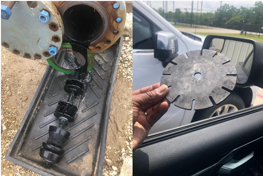
Figure 17--Condition of the 6" Gauge Pig After Being Run Through The Pipeline
