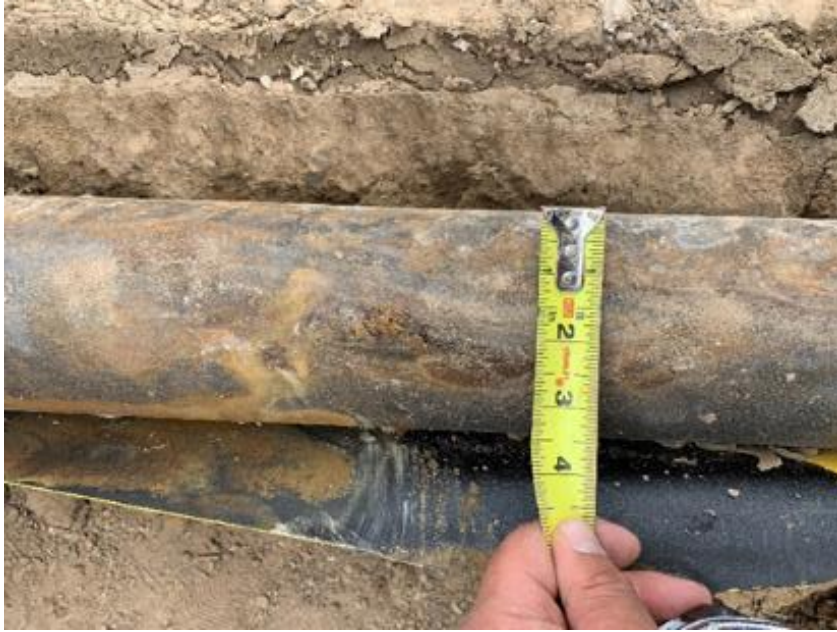
Figure 8 4" Pipe with an OD of 4.5", Showing an Ovality of 1"
