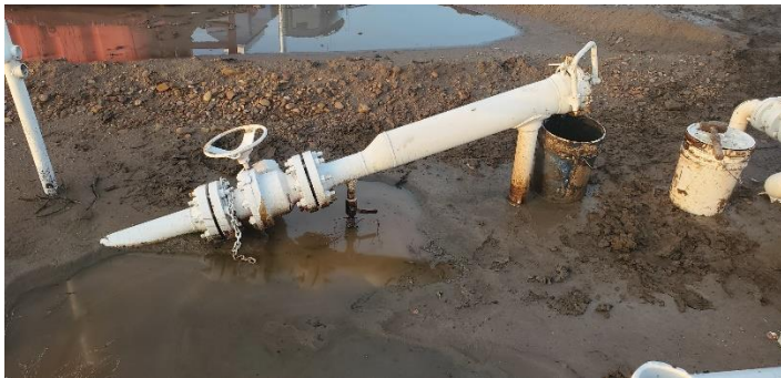
Figure 6--Launcher with Short Oversized Section and No Way to Push Product Behind the ILI Tool
