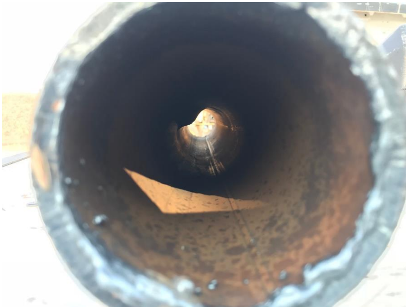
Figure 9--Dent in a 3" pipe
