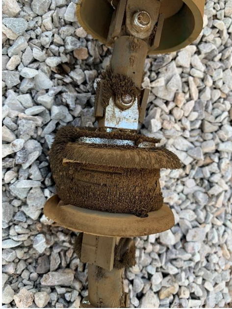
Figure 10--Magnetic Cleaning Pig with Ferrous Debris
