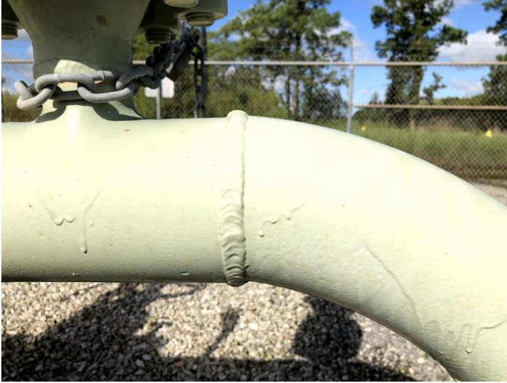
Figure 4--Location of a 3.6" Restriction in a 4" pipe--Sch. 80 Bend and Tee (Note the High/Low Weld)
