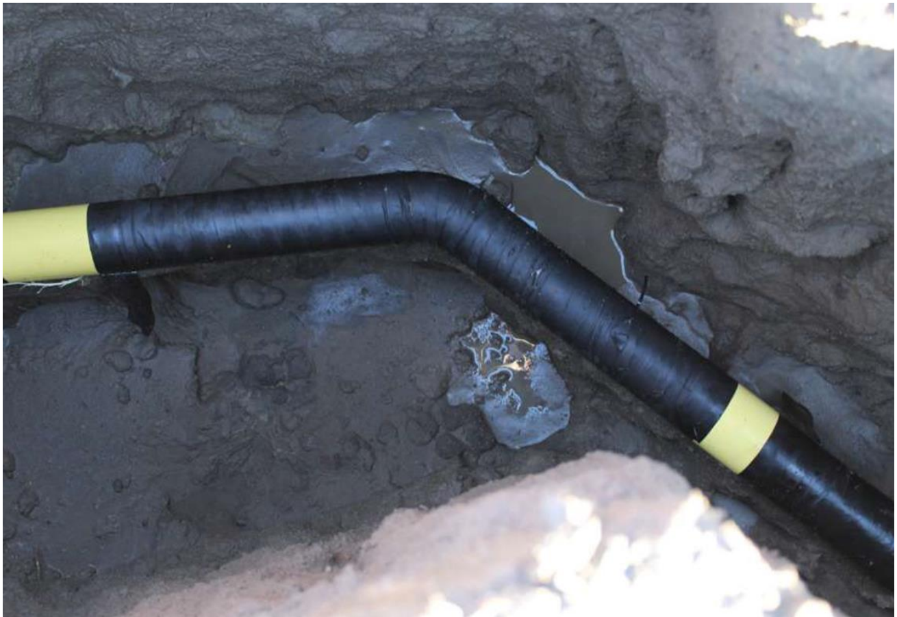
Figure 9 A confirmed 1.5d, 45 deg. bend in the pipeline.
