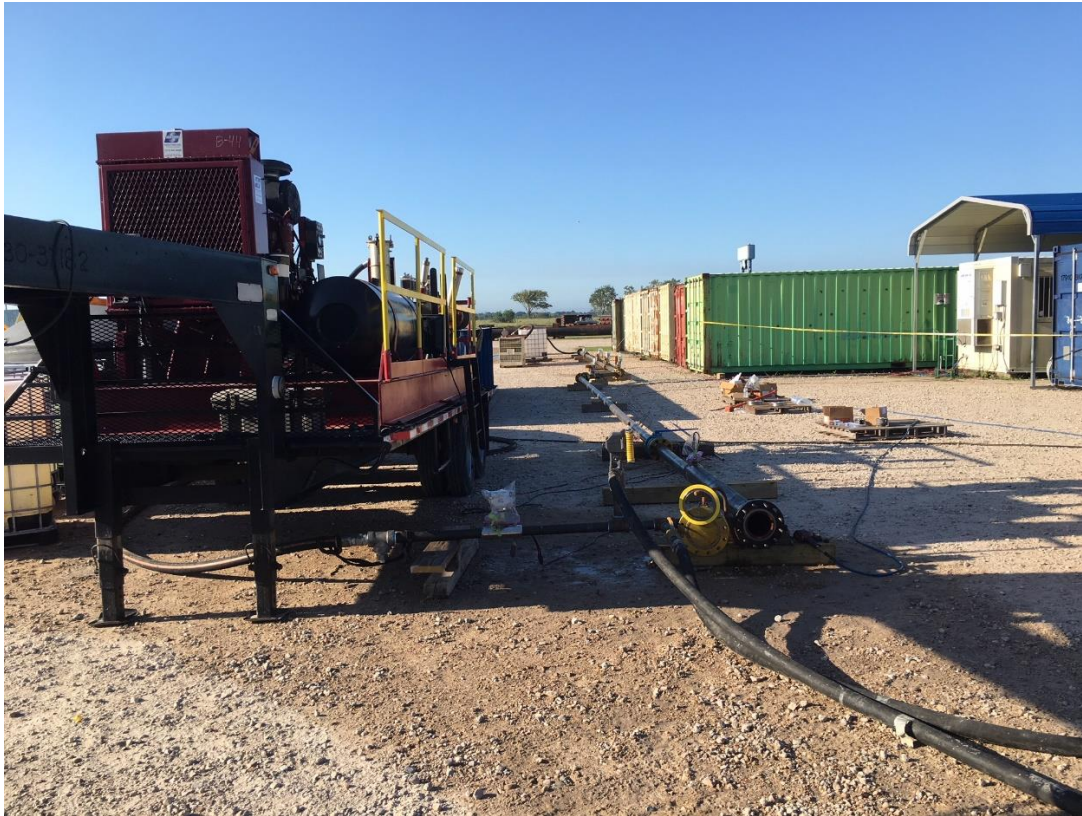
Figure 2 Test Pipe Showing Launcher and Receiver, Bends, and Pump
