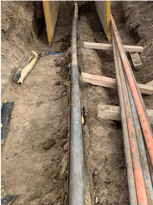
Figure 13 4" pipeline with Fiberoptic Cables in Same Right-Of-Way
