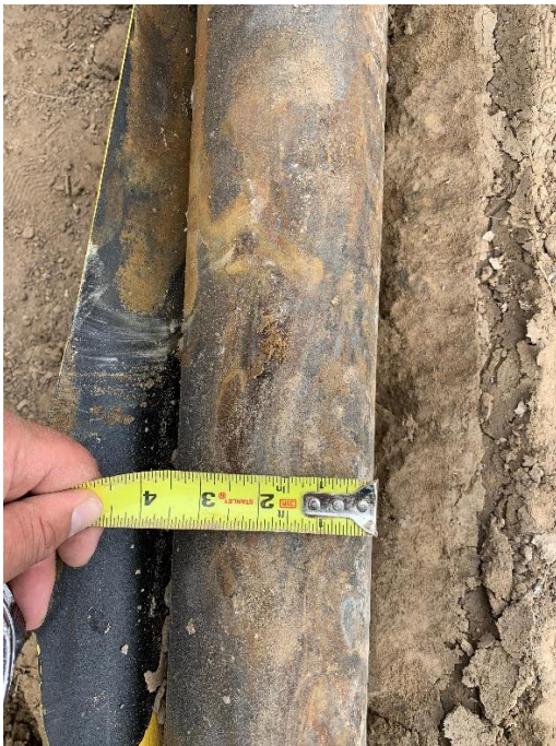
Figure 14 4" Pipeline with an ID of 4.5", Showing an Ovality of 1"
